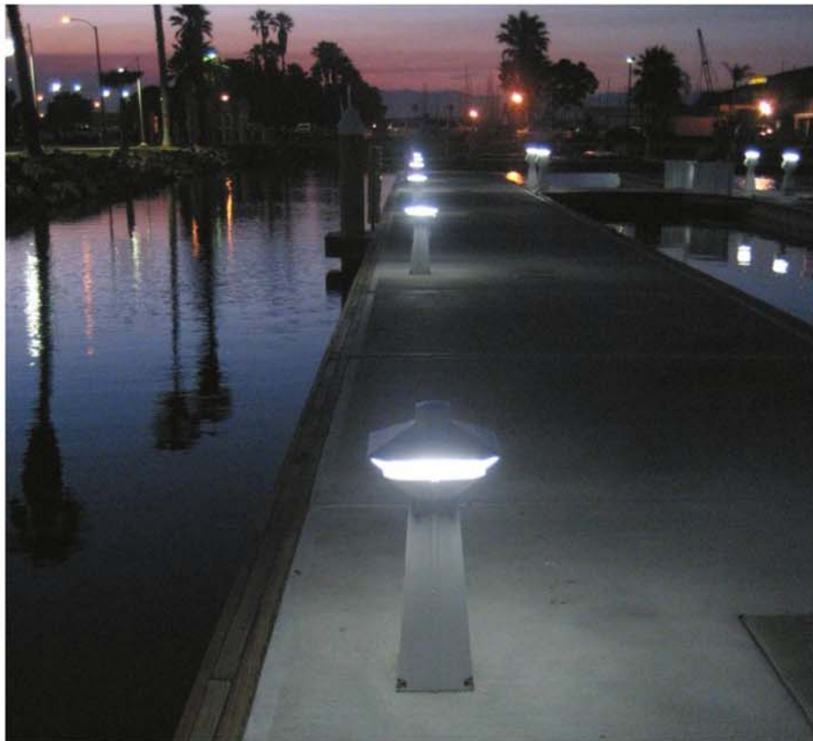
This pedestal lighting at Channel Island Harbor Marina in Oxnard, Calif., reduces the overall power consumption with a low energy LED.
