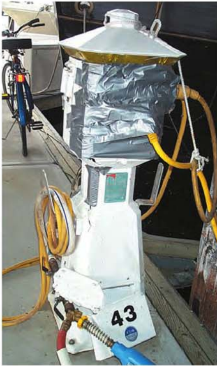
Regular inspections of the electrical system, even a simple dockwalk, will prevent dangerous situations like the one pictured here.
