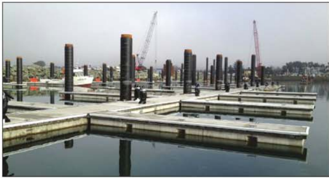
The replacement piling at Crescent City are massive and numerous. They are socketed 35 ft. into the bedrock.
