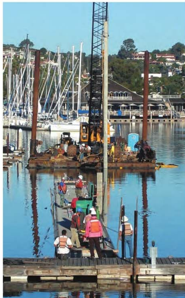
The renovation project at Silver Gate Yacht Club Marina required five boat repositionings. Credit: Bellingham Marine
